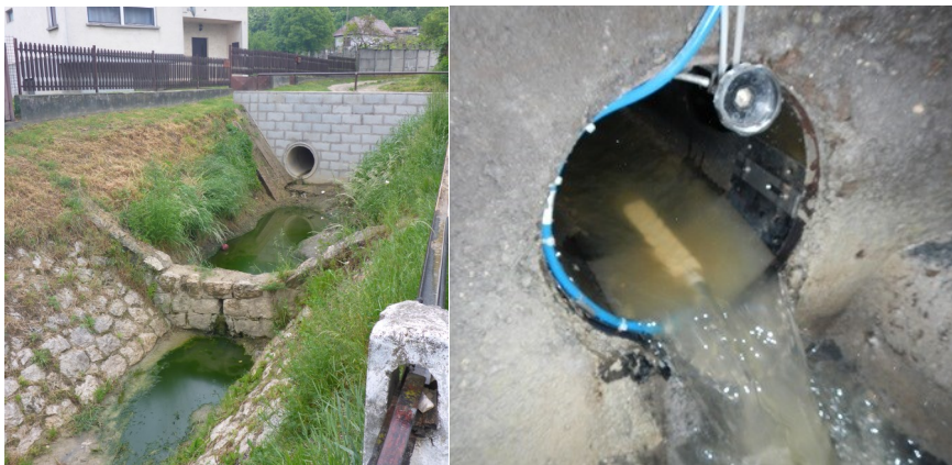
Storm water outlet and sewer manhole © DHI
