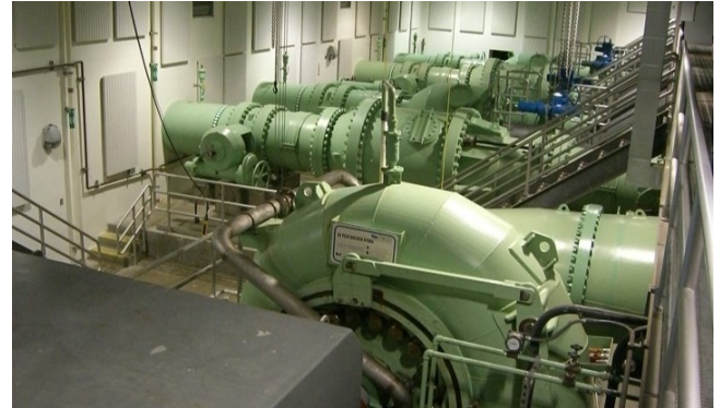
Flow control regulatory station and hydropower facility. © DHI
