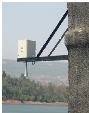
Reservoir water level sensor (RADAR)
